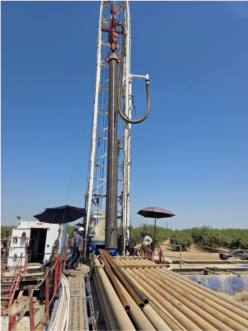
20" Steel Casing, Louvered Section
